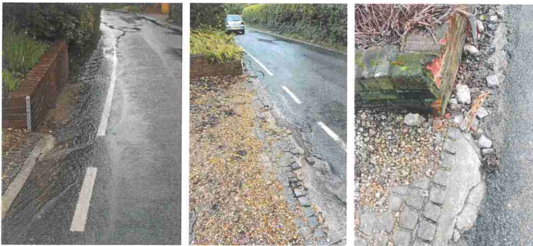
Before, after and later photos of a side wall, with the iron reinforcement first being hit and bent, and then hit again and completely knocked off.
