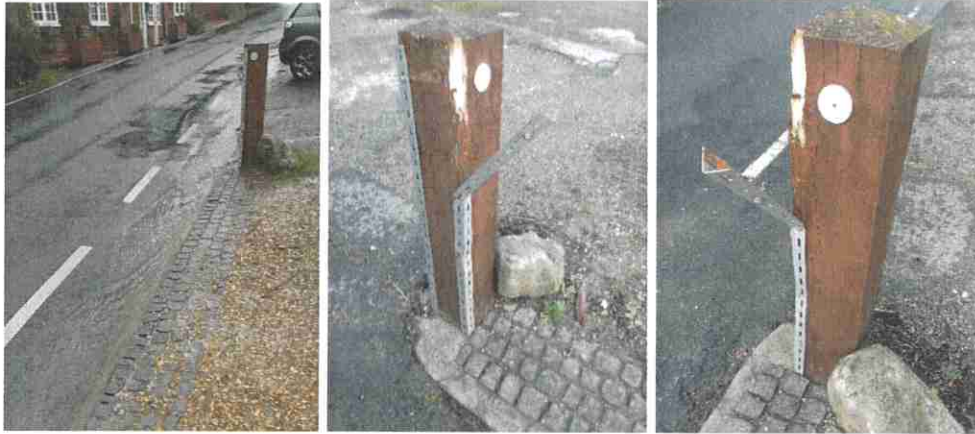
Before and after photos, showing how the 4-inch bolts of an angle-iron reinforcing strip had been ripped from this post on 18 January 2023, bending the iron over. Incidentally, note too the stream of water running down the road.
