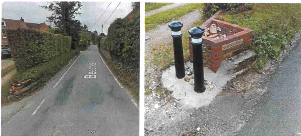
Courtesy of Google's Street View, the first shot shows the damage to another wall, and the second shows the significant remedial measures thought necessary by the resident.
